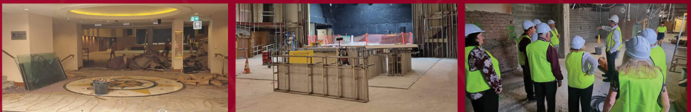
Left-Right: Demolition of the Function Centre foyer; inside the Whitlam Theatre; Revesby Workers' Club directors on a tour of the construction site.
